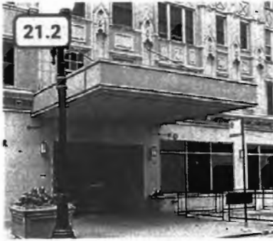
✘ Figure 80. Unacceptable example of a replacement canopy (Bryn Mawr Belle Shore Apartments)
