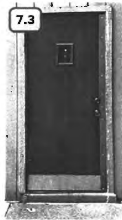
✗ Figure 46. Unacceptable example of a flush door
