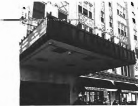
Figure 79. Example of a historic canopy. The adjacent Figure 80 is an unacceptable example of a replacement canopy.
