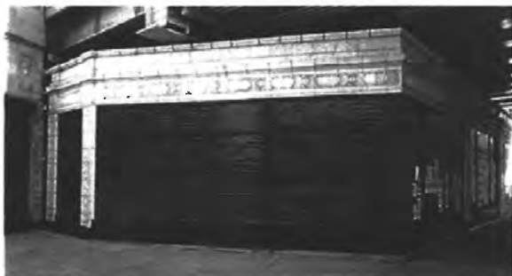
✗ Figure 41. Unacceptable example of a facadectomy as the facade has not been integrated into a new development, but left as an unoccupiable portion of a building and the storefront infilled with brick and a fake storefront frame
