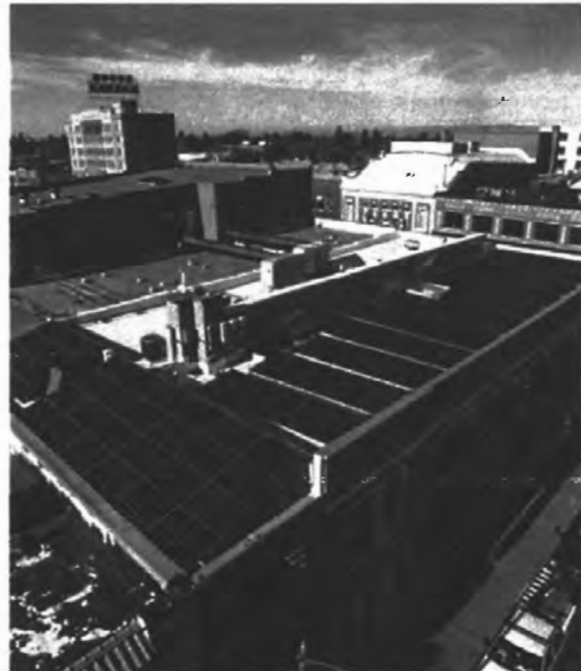
Figure 182. Example of solar devices installed onto a historic commercial building (OnSite Energy, Inc.)
