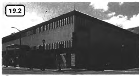
✗ Figure 71. Unacceptable example of materials used at the primary facade
